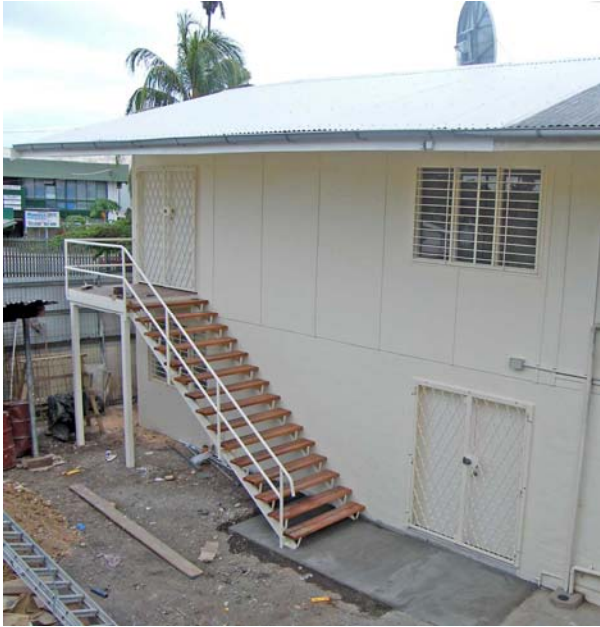
Nov. 6 Stair railing completed, also cement slab, stair's wood is stained, security doors are installed.
