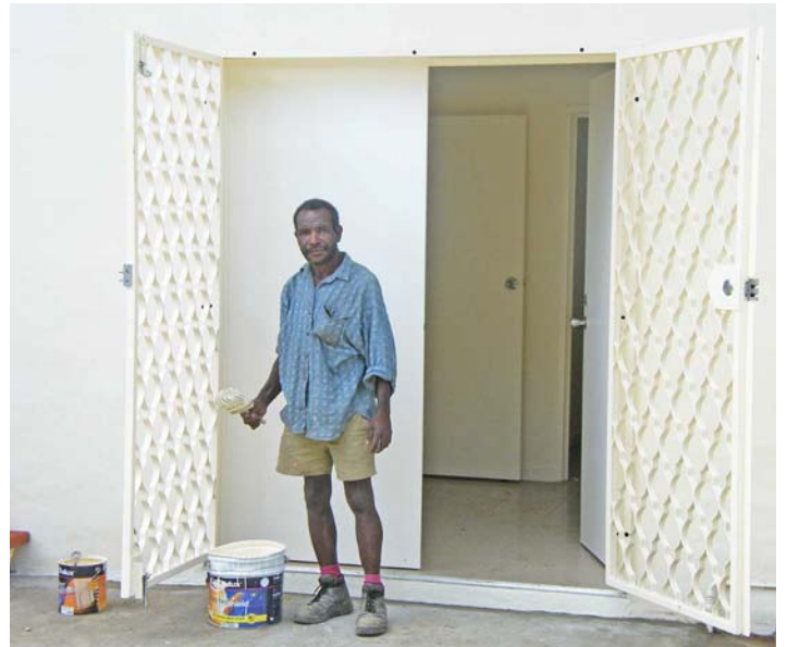
Nov. 10 Final touch-up work is now being done – and ensuring nothing was missed. For example, water has yet to be turned on.
