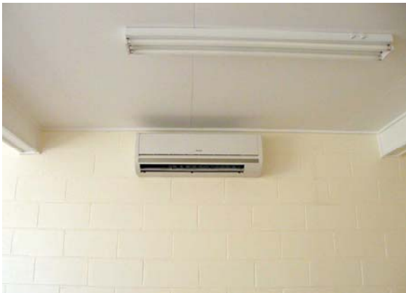
Nov. 10 Downstairs air conditioning is running fine
