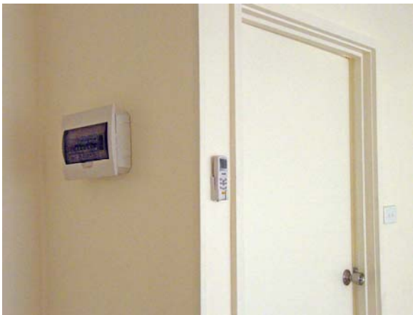
Nov. 10 Final items like fuse box, air con remote control, door knobs, and light switches are all finished
