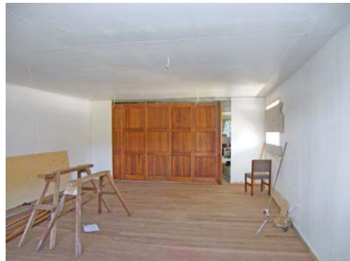
Oct. 18 Upstairs a room divider is installed to either join the original conference room and the new room for large meetings and workshops, or separate the rooms
