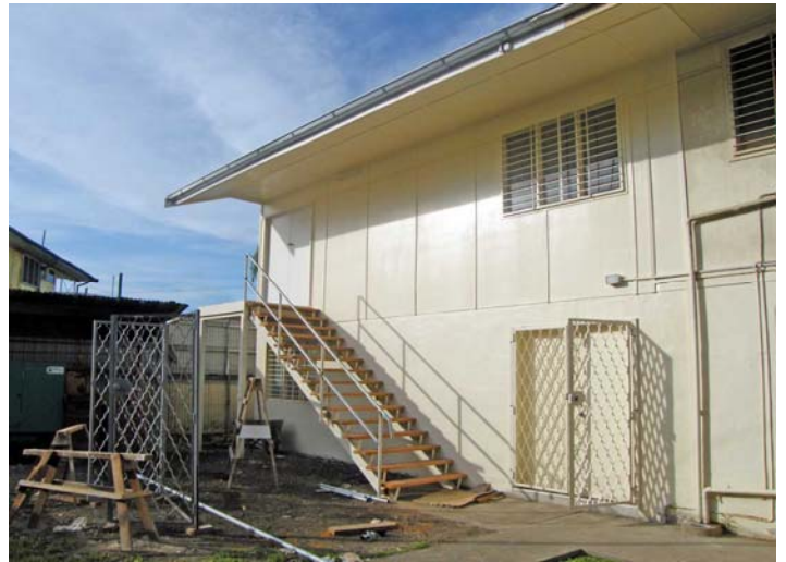
Nov. 3 Security lights, window bars, doors
