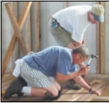
In less than a week most of the hardwood floor was nailed into place at the Owens' house.
