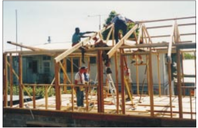
Andrew Likari helps out the World Mission Builders in setting the trusses on the new Multi-Purpose Building.
